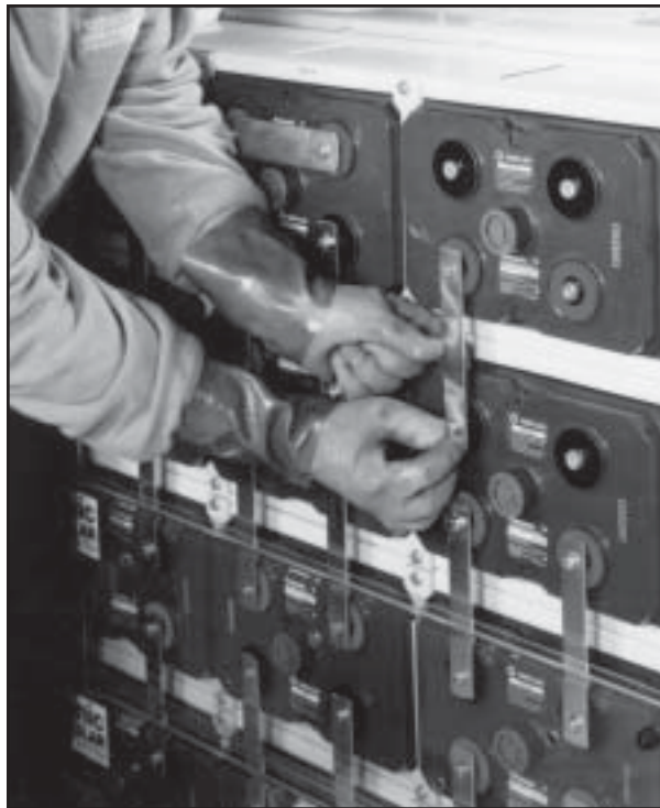
Figure 5.1 Inter-Cell Connectors MSE-1440 Finger Tightening
