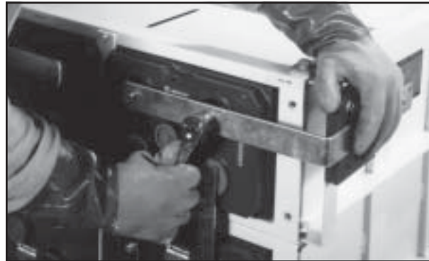
Figure 5.2 Hand Tightening Battery Termination on MSE-500
